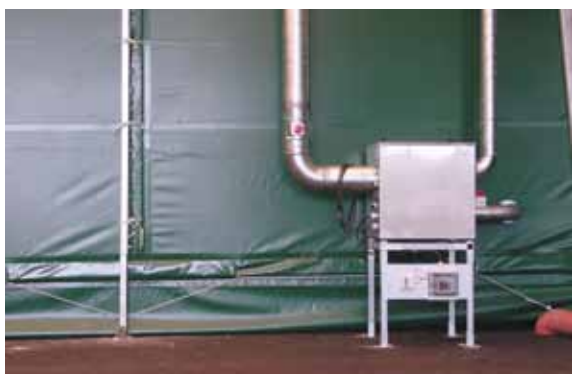
DST dehumidifier Recusorb DR-40 installed in a plastic storage tent.
